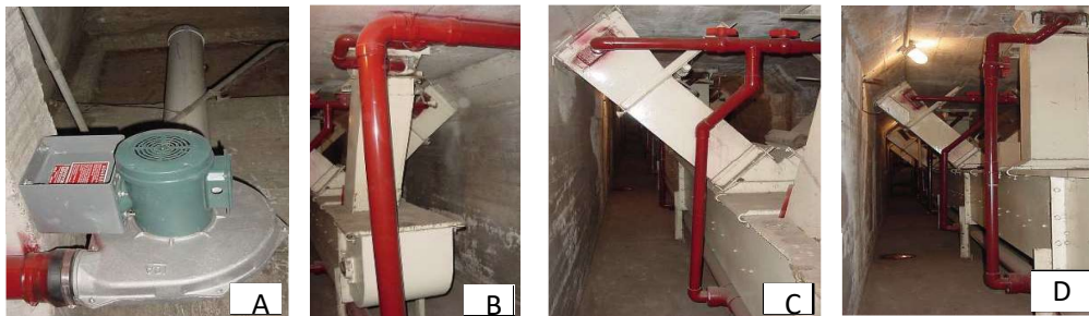
Fig. 8. CLF blower in silo annex (A), pressure manifold (B), lateral pipe to side silos (C), lateral pipe to center silos (D).
