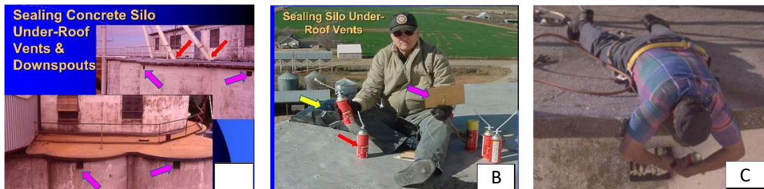
Fig. 6. Foam filling roof deck vents (A), roof vent sealing tools (B), roof vent foam sealing (C).
