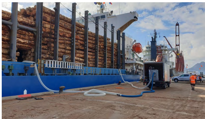
Fig. 2. Setup of the HDS 800, VAPORPH 3 OS ® , and nitrogen cylinders inside a truck and flexible hose connections.
