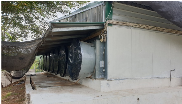
Fig. 4. Sealing of the ventilation fans at the back of the poultry house.
