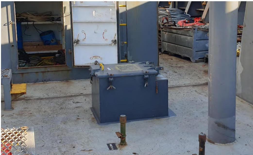
Fig. 6. A manhole cover without a transition piece cover.
