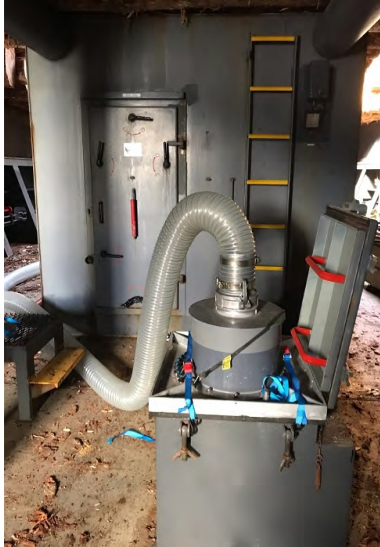
Fig. 5. Close up view of a transition piece cover strapped on top of a manhole.
