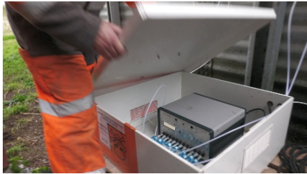
Fig. 6. A PhosCapt®-MP in a cabinet outside the bin.
