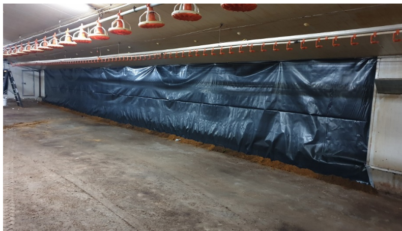
Fig. 5. Sealing of the evaporative cooler (cooling pad) with thick plastic sheet inside the poultry house.
