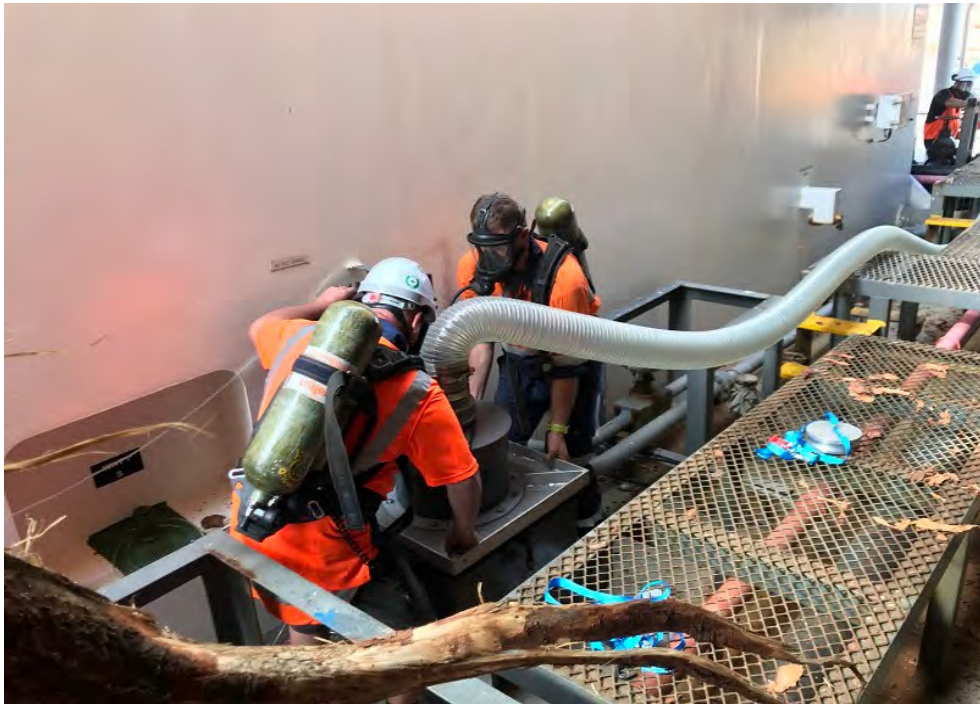
Fig. 4. Setup of a transition piece cover with flexible hose on top of a manhole.
